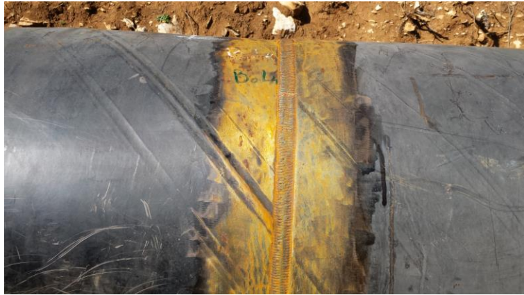
Figure 8. Welded joint in HPP Ternove
